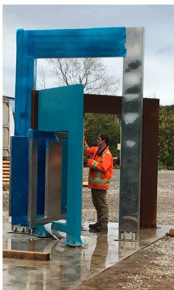
The upright stainless steel section of the sculpture demonstrates undesirable "canning" undulations on the surface of the metal.
