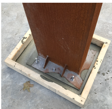
This is the trough constructed at the base of the Corten steel sections of the artwork to capture any bleed from the rust patinated surface of the sculpture. The trough was filled with red pea-shingle as a design aesthetic and method of capturing rust- bleed into an attractive and controlled surface.
